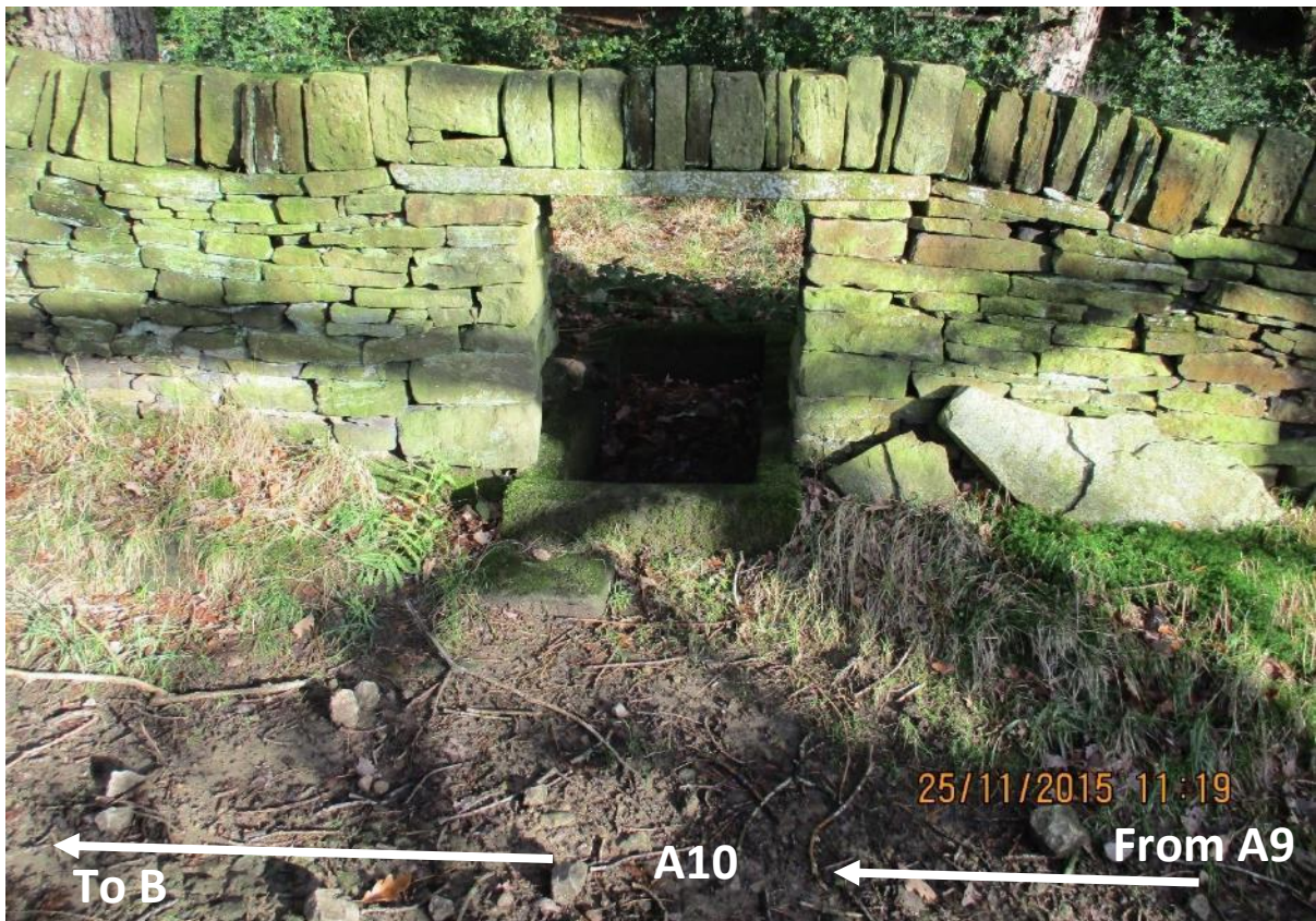
33. Spring-fed trough in wall adjacent to Meltham 70 at point A10. This is south of the remains of buildings at Lower Cote Farm. 25 Nov 2015.
