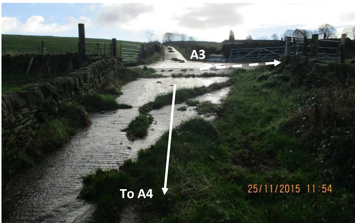
16. View north along Meltham 70 from just south of point A3 (junction with track to Manor Farm). The concrete surface continues for some distance south of the camera position over part of the width of the track to a field gateway at point A5. 25 Nov 2015.
